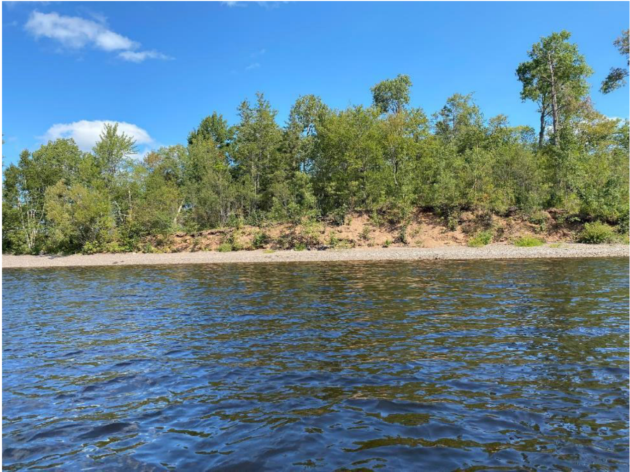
FIGURE 19. SITE #7 FROM THE 2022 GILE FLOWAGE SHORELINE STABILITY ASSESSMENT.
